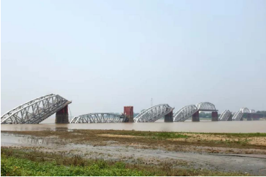
The collapsed Ava Bridge in Mandalay [EPA]
